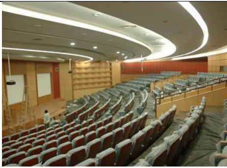
IIT CONVENTION CENTRE, POWAI. ELECTRICAL WORKS OF INDOOR /OUTDOOR SPORTS UTILITY AS IITBOMBAY-POWAI
